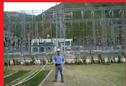
Figure 3. EnerSur hydroelectric plant
