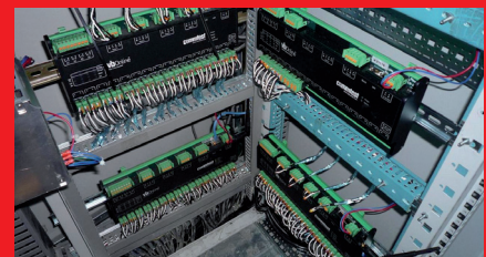
Figure 2. Integrating Commtest's vbOnline and Bently Nevada TM 3500 systems
